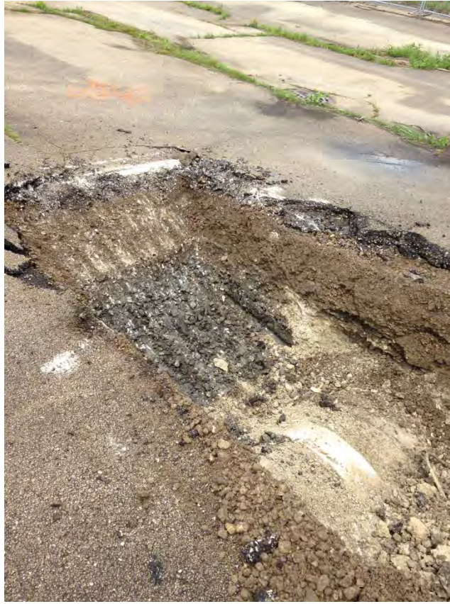
Photograph No. 17 – Concrete Pipe Obstruction at DC-4
