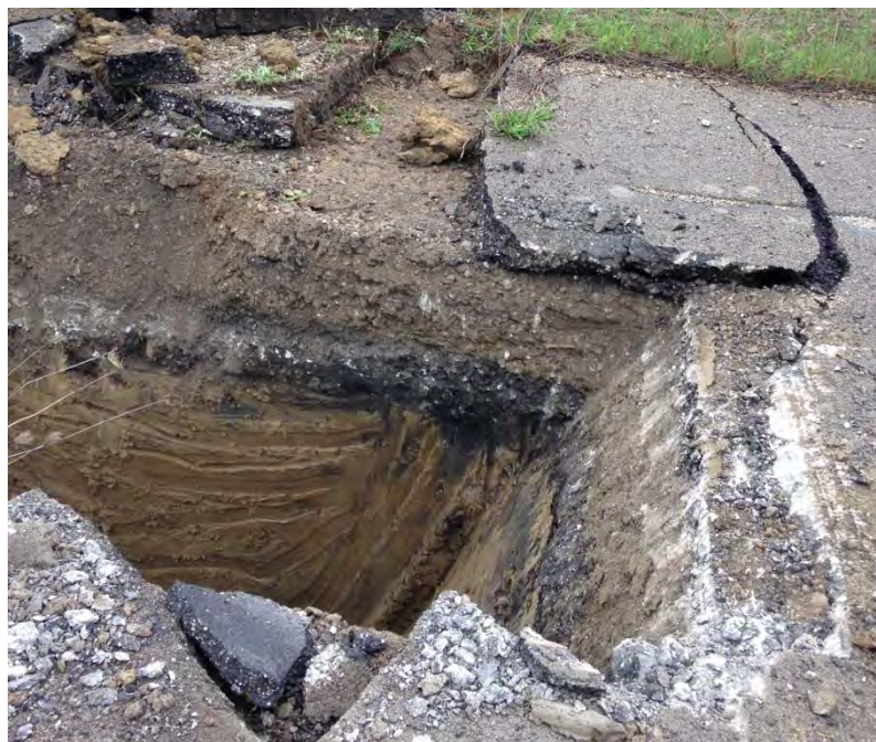
Photograph No. 3 – LT-2 Side View
