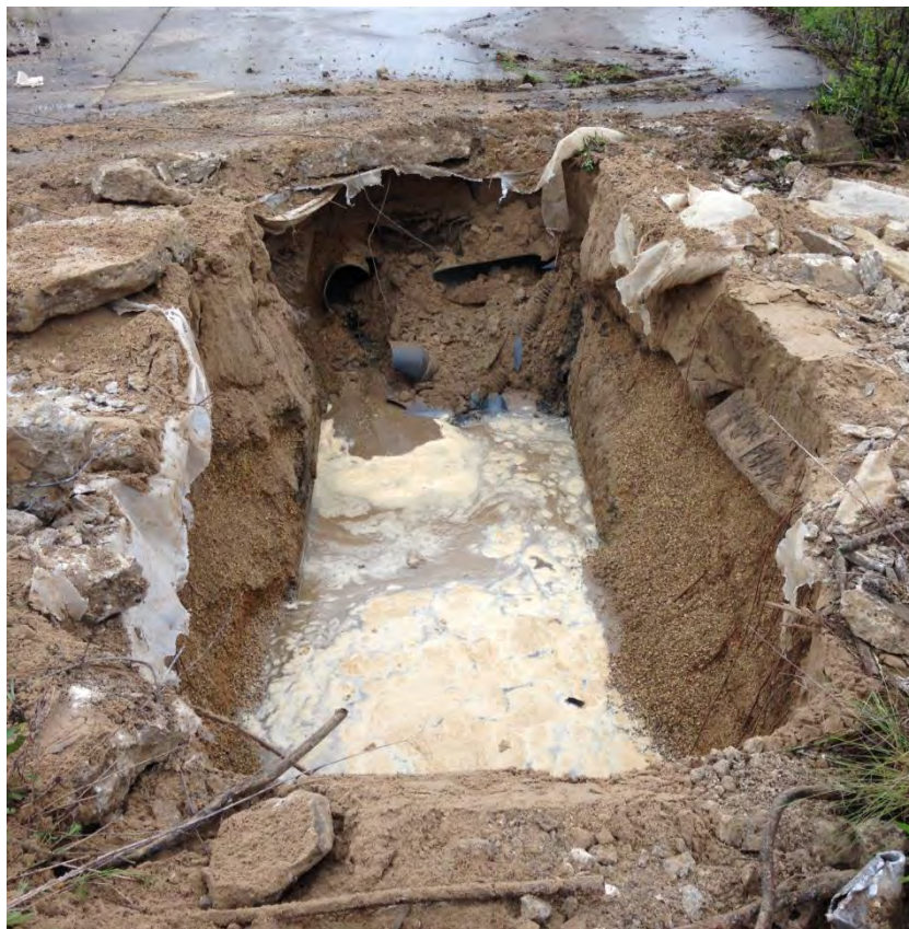
Photograph No. 6 – LT-4 Filled with Water
